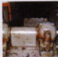
Mechanical: Overheating bearing at pulley end
